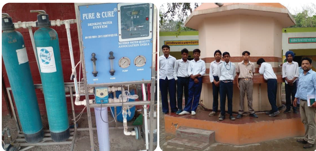
PFC installed RO water plant at Government Senior Secondary School - Jeevan Mall
