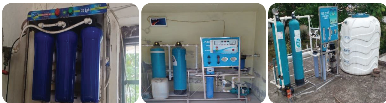
PFC installed RO plants at various Government schools in Ferozepur District
