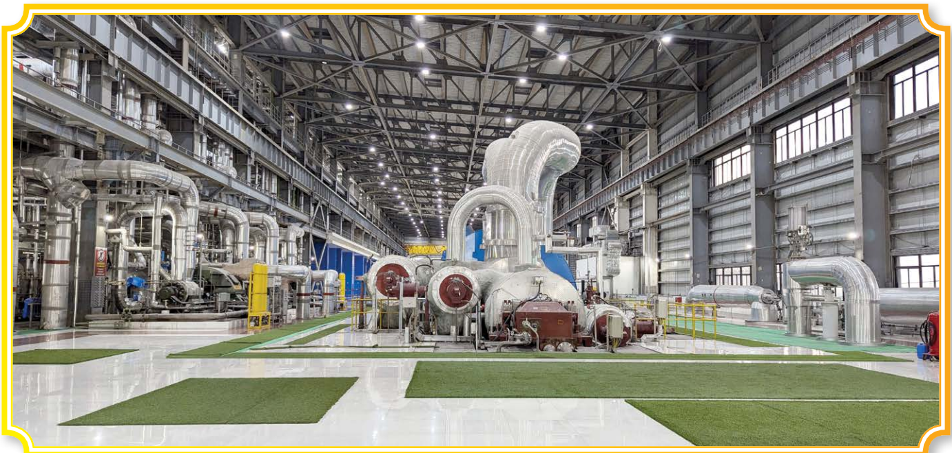
Turbine-Generator of (2X800MW) Adani Power Jharkhand Limited, Godda, Jharkhand financed by REC
