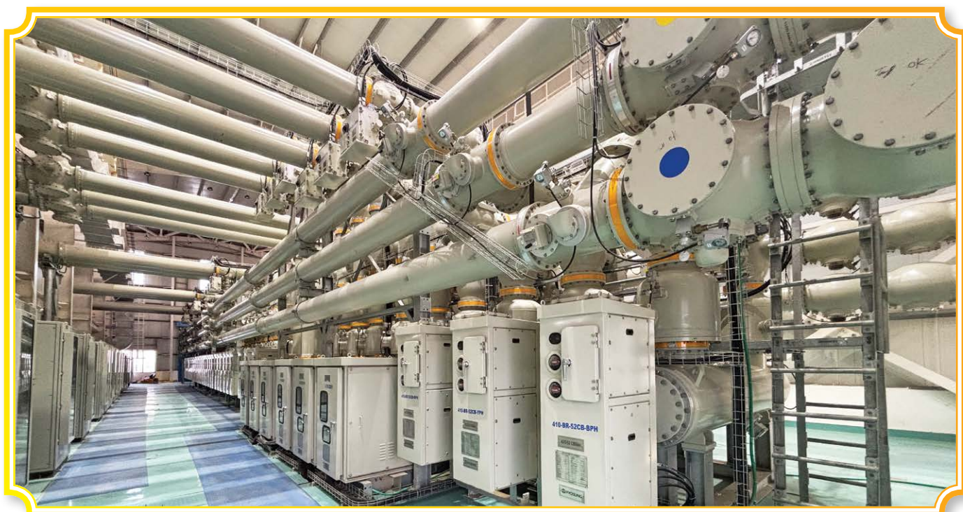
GIS Substation of Khavda - Bhuj Transmission Ltd. (Gujarat) financed by REC
